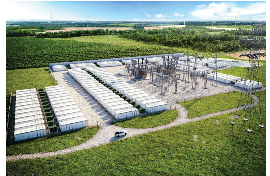
Oneida Battery Storage
