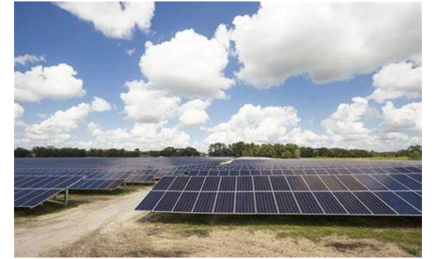
A NextEra solar facility in Lambton County, ON
