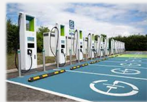
High Power Public Charging Stations
